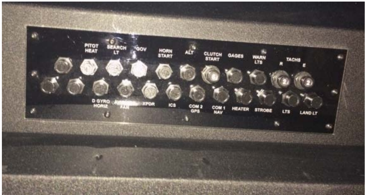
Fig 9: Circuit Breaker Panel
